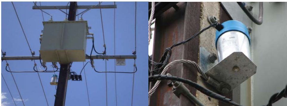
Illustration: Typical LV Capacitor and Street Transformer
