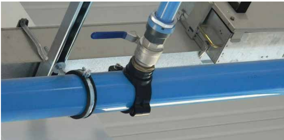
Typical Application for Saddle Branch
