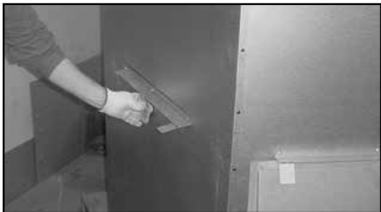
Figure 3.6 Bend Refractory Brackets Back Down
