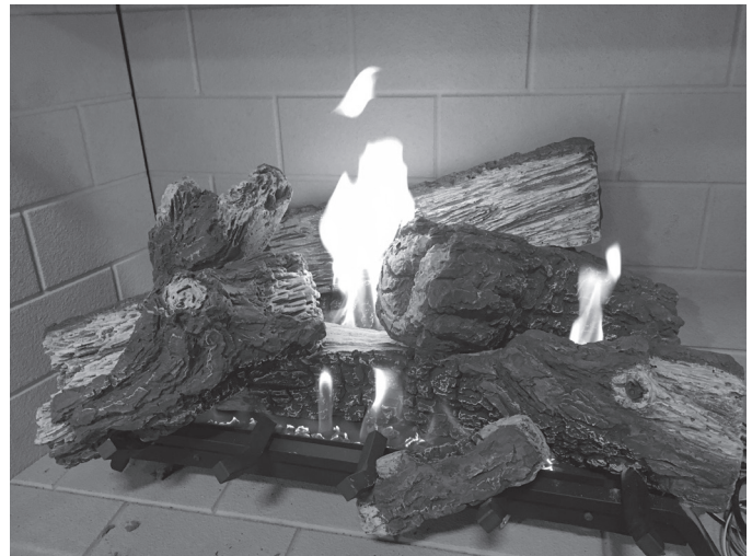
Figure 5.13 - Correct Appearance of Rear Flames
