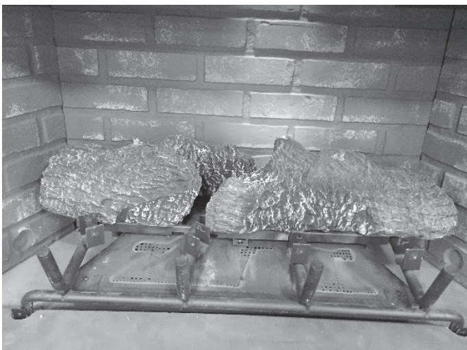
Figure 14.8 Left and Right Rear Log Placement
