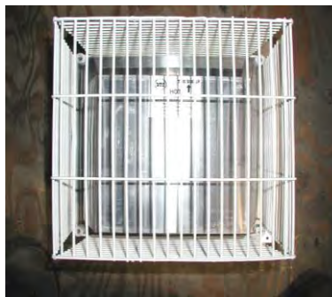
VIEW OF SAFETY CAGE
