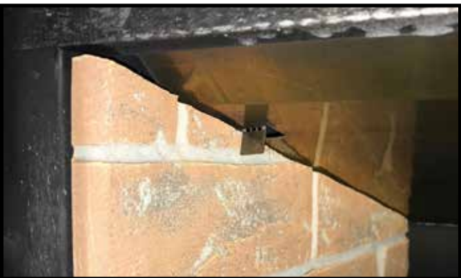
Figure 6 Left Refractory Handbend Tab
