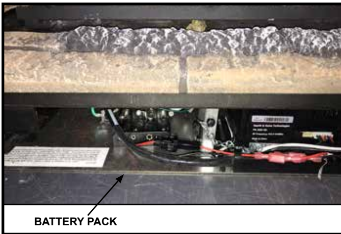
Figure 6.3 Battery Pack Installed
