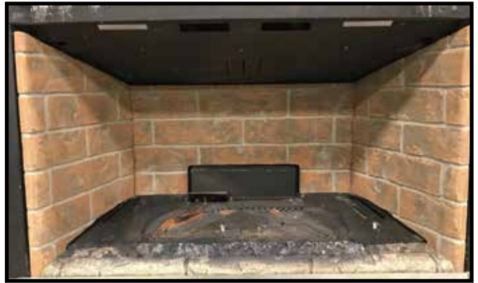
Figure 8 Refractory Kit Installed
