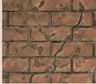
Fire Cracked Brick
