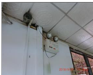
Photo of fire safety equipment Emergency light.JPG
