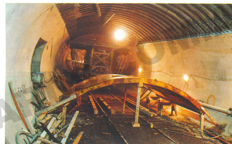
(Above left) For the Caulfield connection in the Caulfield-Sandringham loop, the box section tunnel and ramp were 60% complete at the end of the year.
