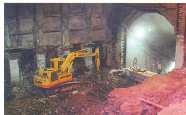
(Left) Activity directed to the completion of the Y-junction of the Clifton Hill loop and City Circle.
