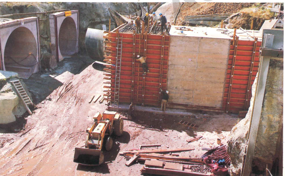
Box section tunnels are built by "cut and cover" under operating railway tracks. Circular tunnels which run under city streets are constructed by mining methods. A special collar links them. (Below) Two views of the transition from box tunnels to circular tunnels near Adderley Street.
