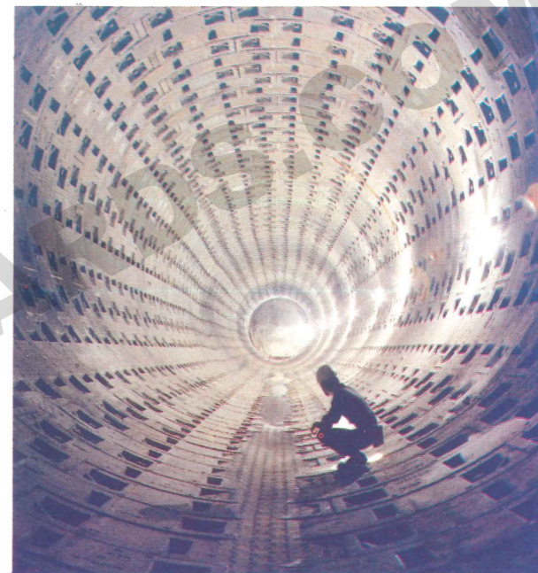
(Above) A breakthrough at Flagstaff Station in the Burnley loop tunnel provided the first opening for the full length of one of the four loops around Melbourne.
