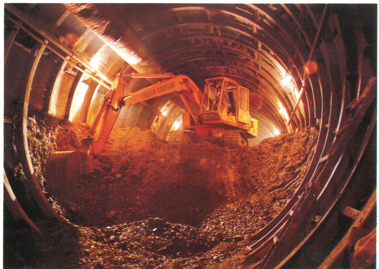
(Below) Bench excavation in a running tunnel using a tracked back-hoe. About 90% of tunnel excavation had been completed by the end of the 1977/78 year.
