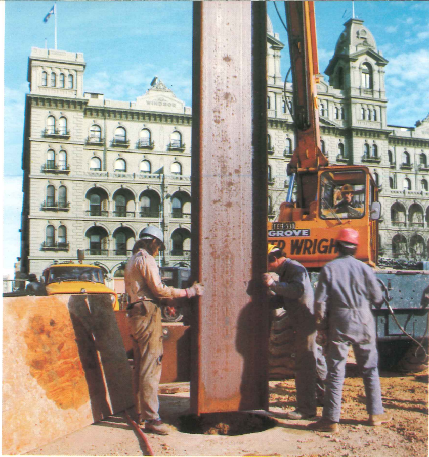
Parliament Station is steadily taking shape under Spring Street near Parliament House. During the year work was begun on construction of a booking hall for the southern entrance of the station. (Left) Pile installation opposite the Hotel Windsor. (Below) A temporary rail track provides access for a work train to a station platform area.
