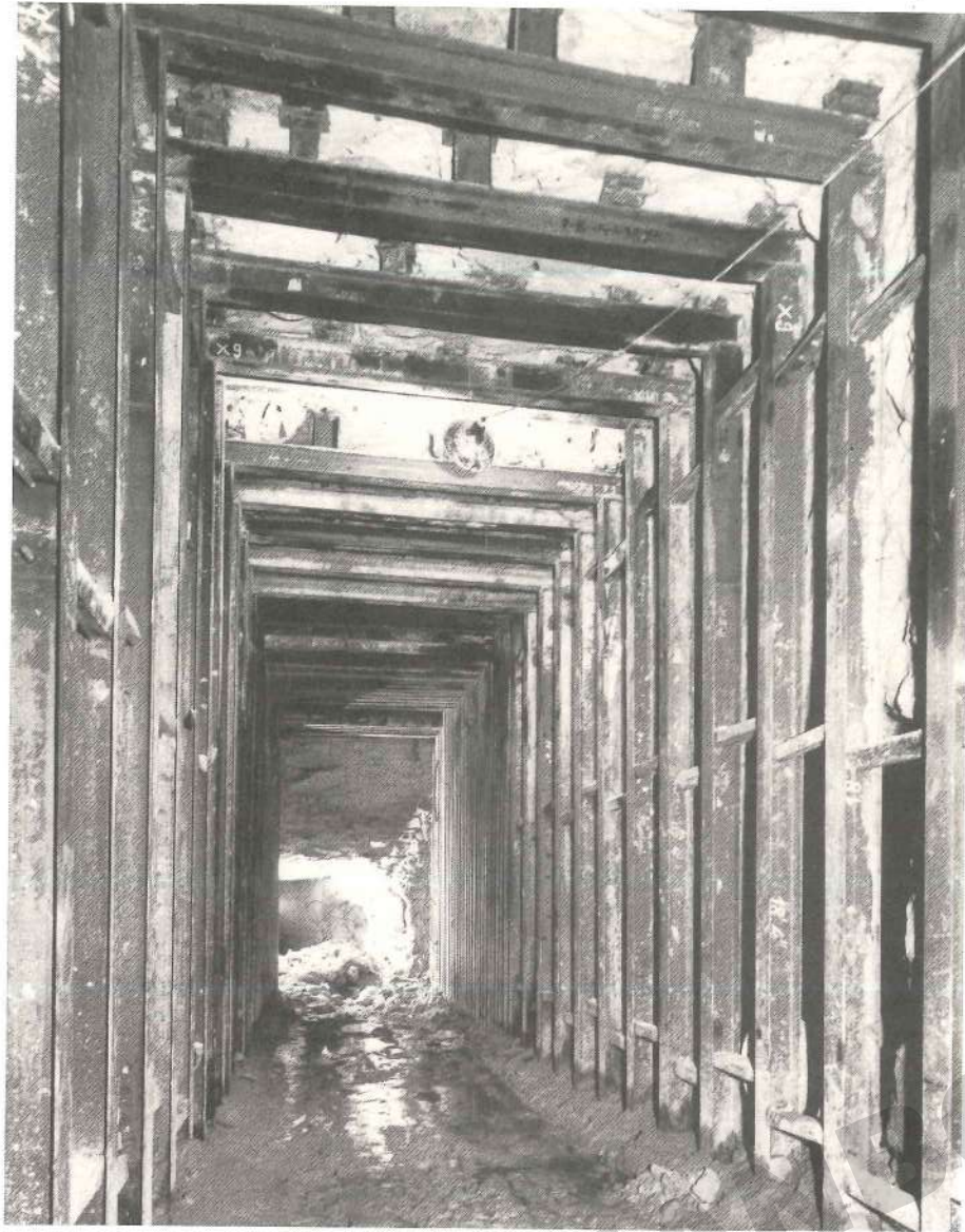
Stazione di Martin Place - armature provvisorie Martin Place station - up column drive - Temporary Steel supports under existing tunnels
