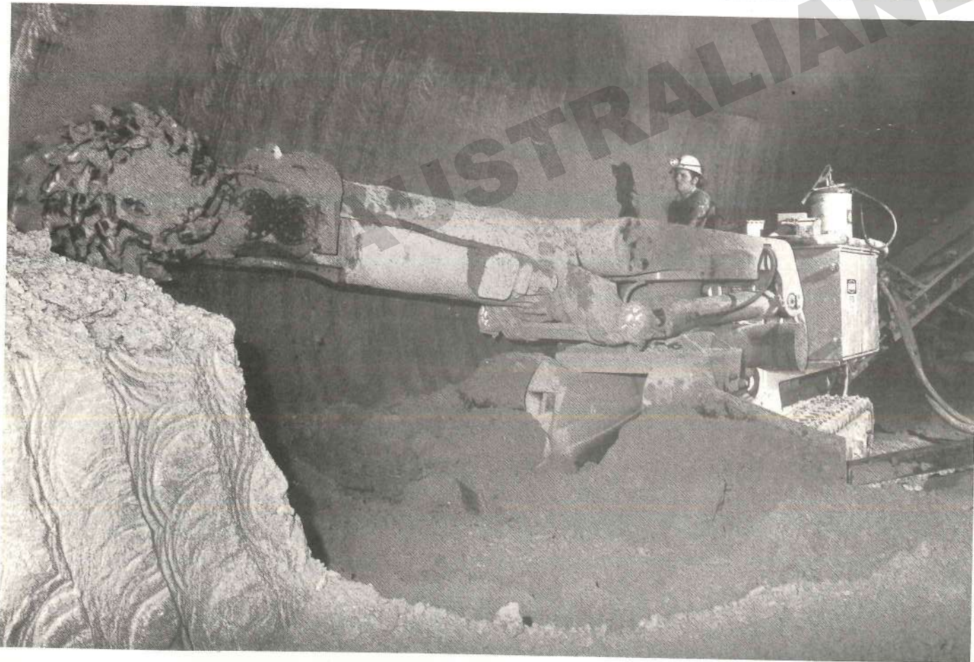
Excavation of the bottom bench of the tunnel with an Alpine Road- header
