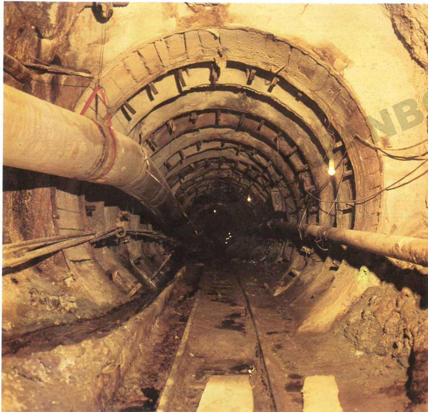
Digging through chemically treated ground on the Paola side of the tunnel
