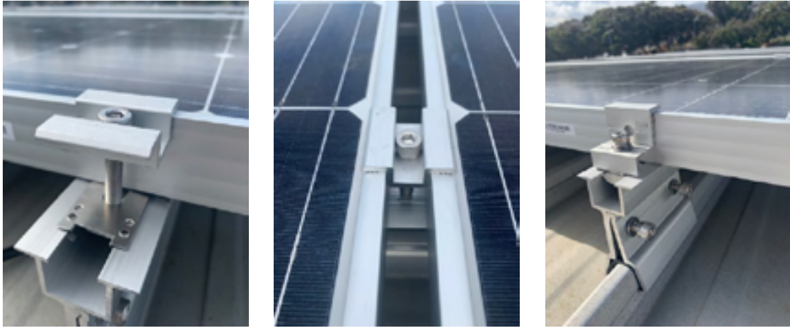
Figure 2 ASCENT Kliplok mounting using the mid clamp to clamp 2 panels, and the end clamp to clamp the panels at the end of a string
