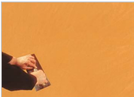
Step 5 - When the product begins to dry, proceed with compacting and polishing the wall.
