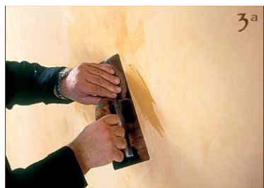
Step 7 - At this point the product will penetrate into every little crack and with slight pressure the surface will be perfectly smooth. We apply... and remove Spatula Stuhhi for about 1 square meter and ...
