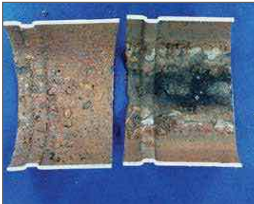
Untreated Steel FPS Pipe
