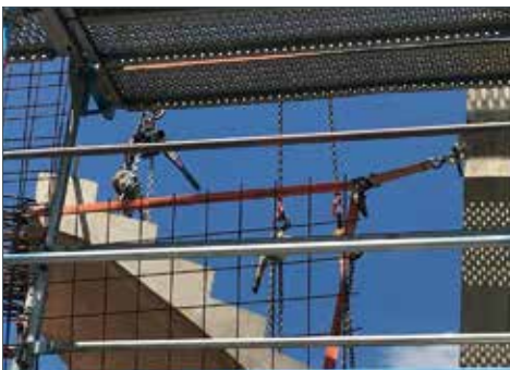
Positioning of loads Especially when using multi-fall chain slings (e.g. installation of stair segments and turbines)
