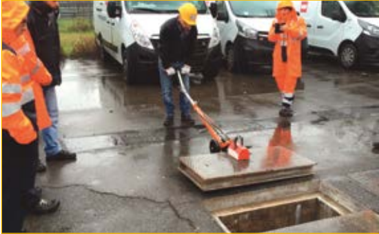
Uso 1: necessary use in the presence of manhole covers excessively heavy or worn out.
