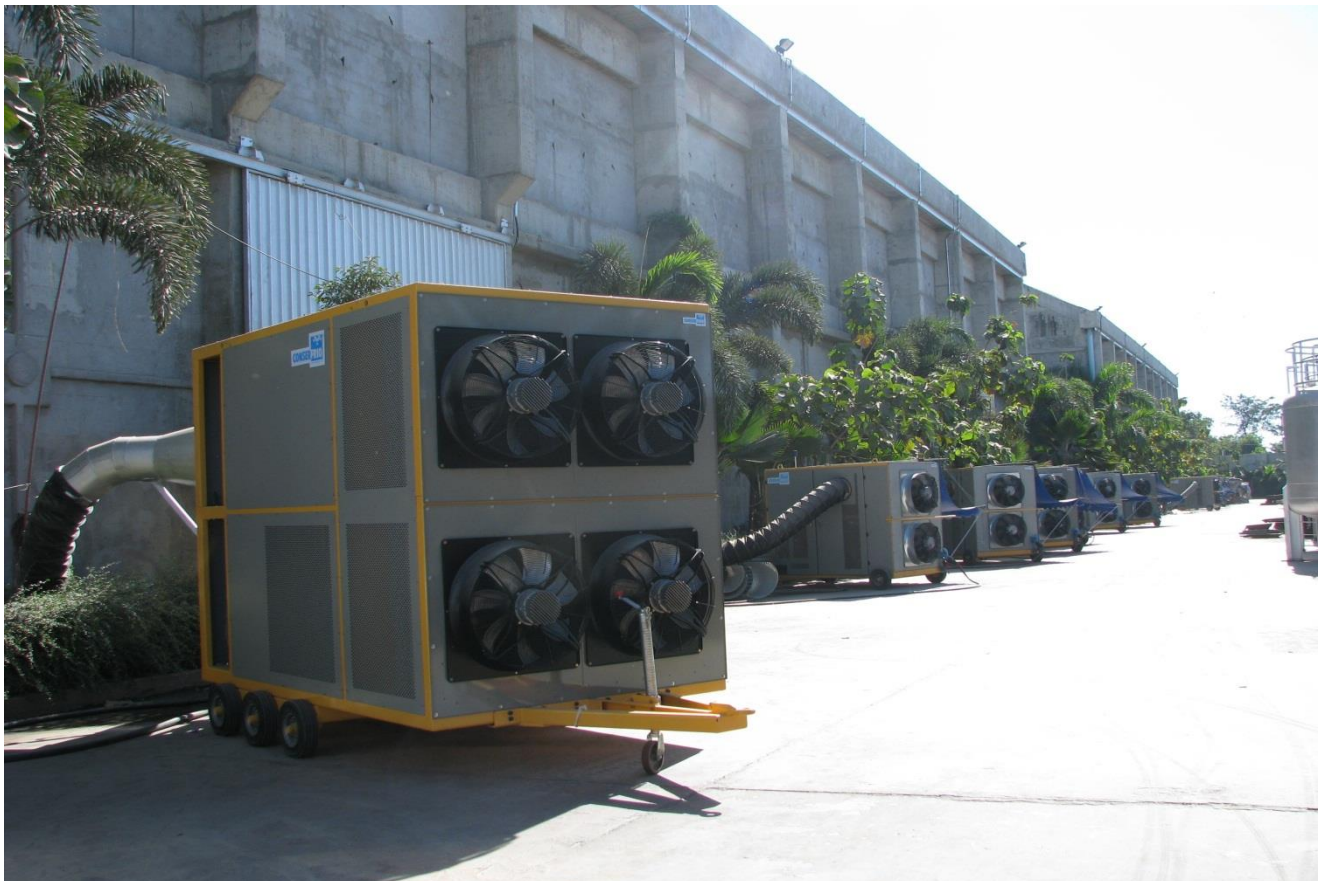
1 unit F450TD chilling grain stored in a warehouse
