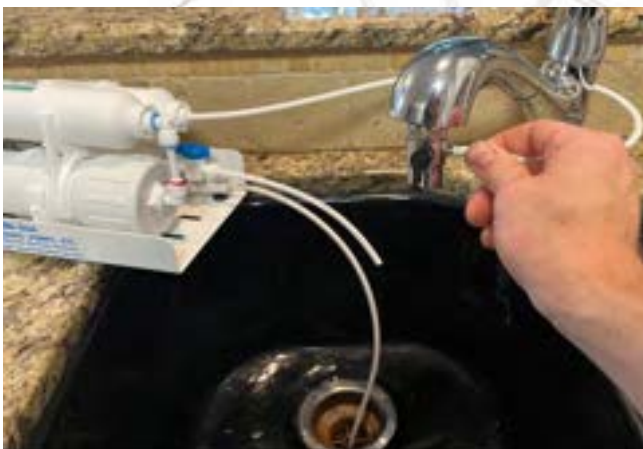
The picture above shows an example of a fully installed Mighty Mite RO System.
