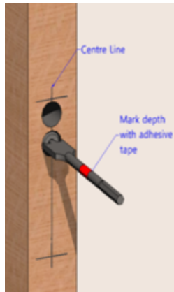
Fig 2 Mark a centre line* between the marked lock case lines. Drill a series of 19mm diameter holes a little deeper than the lock depth. Do not drill above or below lock case lines. *For doors more than 50mm thick, mark an offset line
