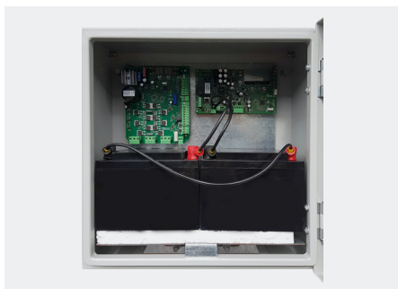
Inside the Power Box
