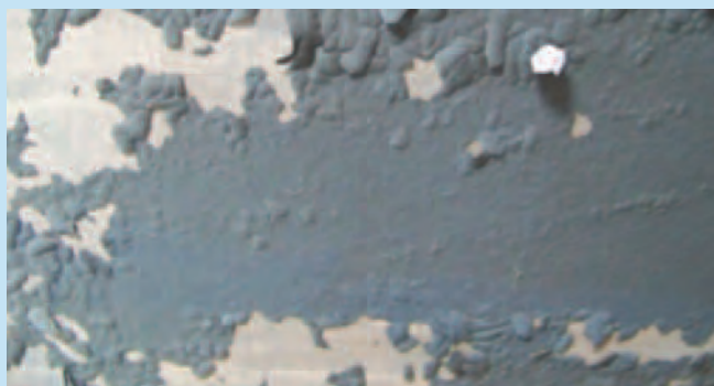
Detachment: The time window was missed between the no-sand primer and the antifouling paint.
