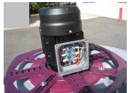
18. Do the correct wiring between the switch and the motor, respecting tension.
