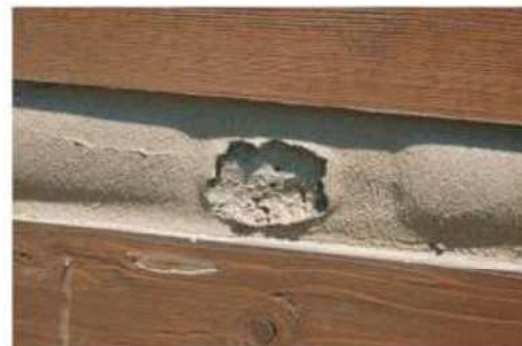
Blister formed by trapped air or applied in hot sunlight
