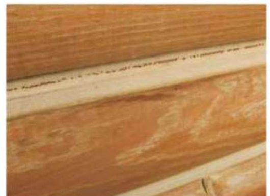
Chinking applied too thin, must cut out and replace
