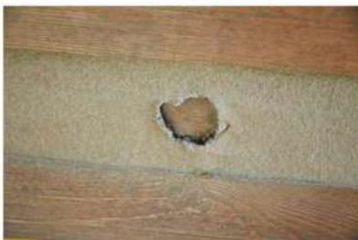
Blister formed when thin layer applied over improper (in this case, none) backing
