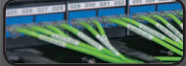
Patch Panel / Block-66 Labels
