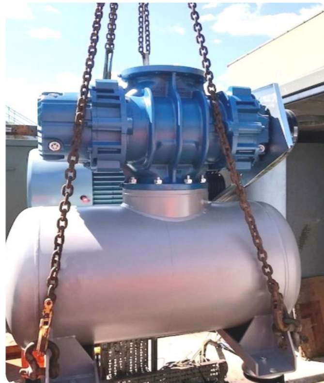
Above: Veolia Newbridge installation
