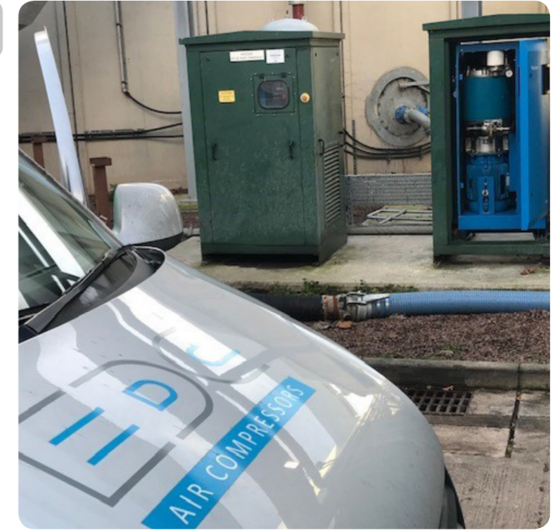
Above: A Hydrovane overhaul
