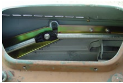
Fig 9: A view of the left pivot shaft, cross link and first link through the gauge cluster opening.
