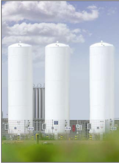
AC SCS.1 Line Vertikal Bulk Tanks
