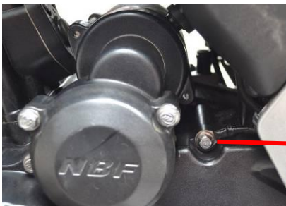
GOUNDED CABLE TO ENGINE HOUSING
