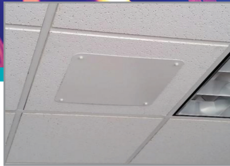
■ Installed Condition: PSIBVHF and PSIBVU78
