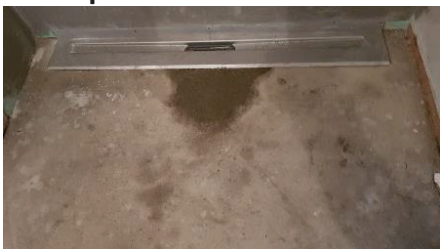
Level the floor with screed taking into account the thickness of the UniSlope Board plus 2mm of tile adhesive.
