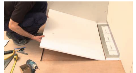
Screw the UniSlope board and end fillers into position using dry wall screws.
