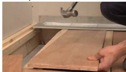
Cut the ply wood and place on top of the battens between the joists.
