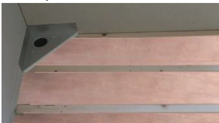
Cut the ply wood and place on top of the battens between the joists.
