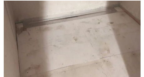
Place the UniSlope board and end fillers into position and screw down.
