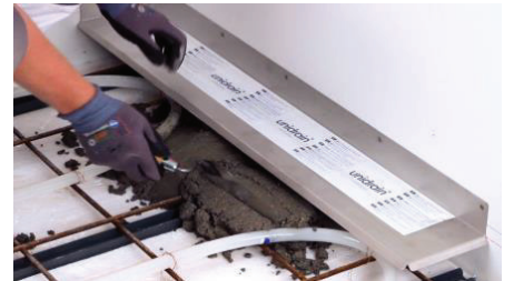
Pack the outlet and underside of the drain with screed making sure there are no air pockets.
