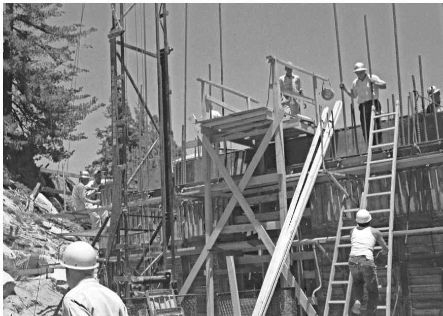
Palm Springs Aerial Tramway construction in 1963. PHOTOS PROVIDED BY THE PALM SPRINGS HISTORICAL SOCIETY
