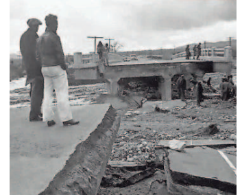
Damage to the bridge on South Palm Canyon Drive in 1938.
