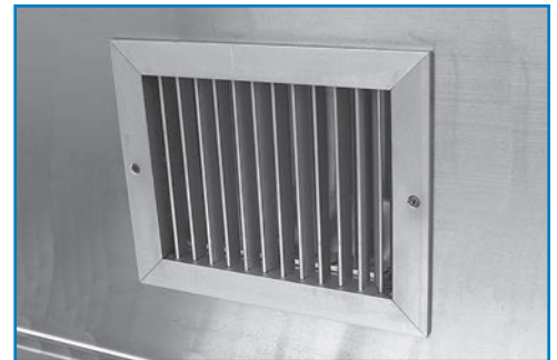
OA-206 - EXHAUST DUCT 8 x 10, Each
