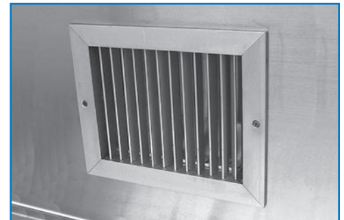
OA-206 - EXHAUST DUCT 8 x 10, Each
