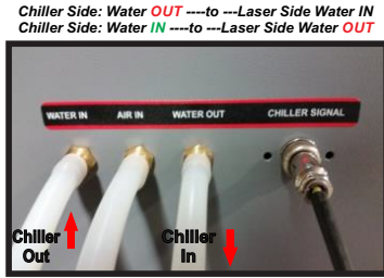
Chiller Side: Water OUT ---to ---Laser Side Water IN Chiller Side: Water IN ---to ---Laser Side Water OUT Use a Small Heat Gun or Hair Dryer to Soften Hose to get them to Fit onto the Barbed Outlets
