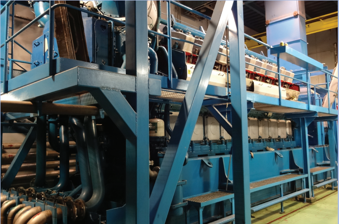
Full circle: The site's 6 MW gas engine
