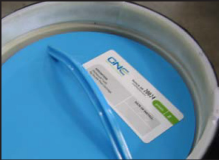
A filter this high is not installed properly.
