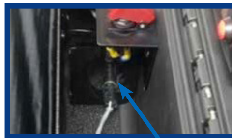
Figure 22. Reconnect Electrical Connector
