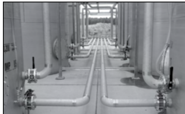
Fig 22 - Fill and discharge tubes
