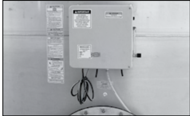
Fig 13 - Airmix liquid fluidizer control box
