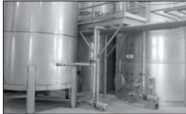
Fig 20 - Permanent fill and discharge system
