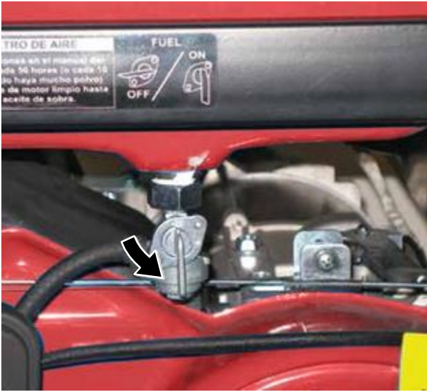
Figure 17 – Fuel Shutoff Valve in the ON Position
