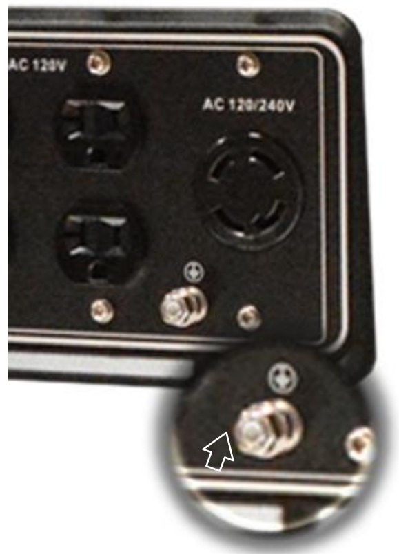
Figure 12 – Ground Terminal on the Control Panel
