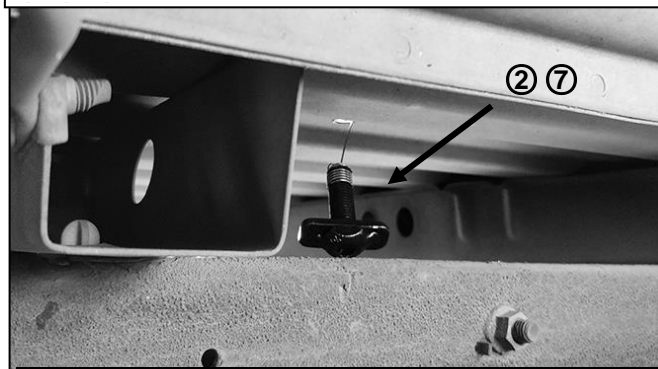
(Fig 3) Thread (1) 12mm T-Bolt into (1) 12mm Fish Wire. Slide the end of the Fish Wire into the drilled-out hole from the bottom of the bed
