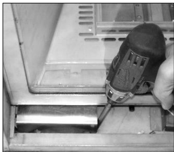
Power Vent Control Module Mounted inside fireplace.
