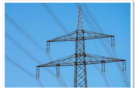
Redirect energy to the grid
