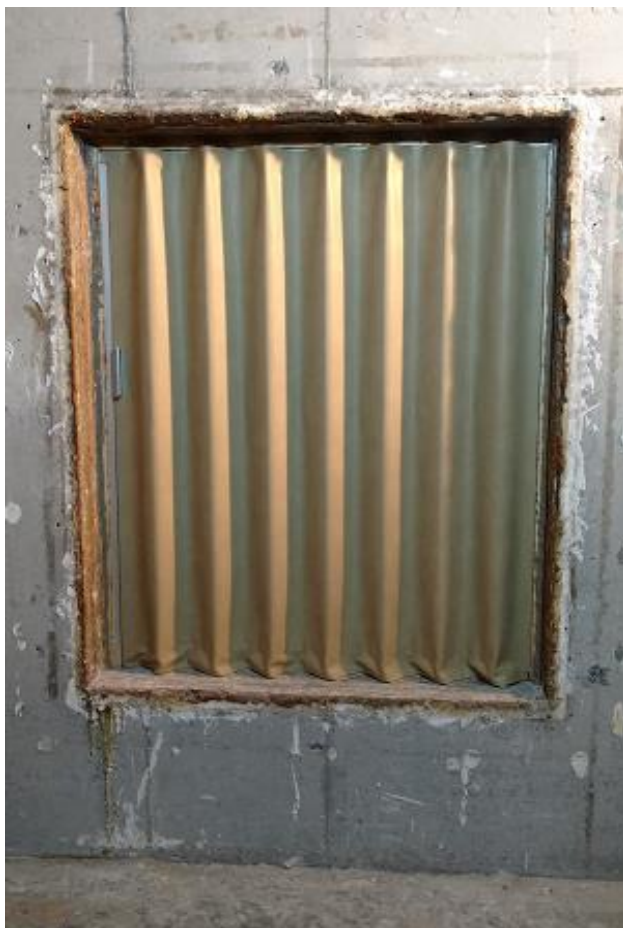
view in Sending Room side
