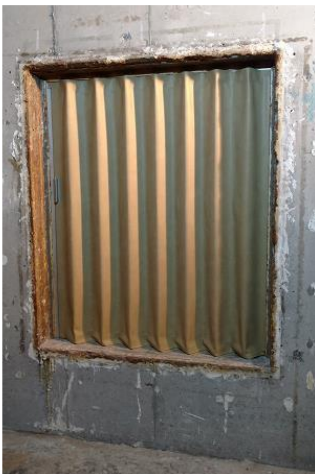
view in Sending Room side
