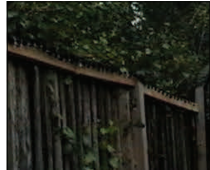
Cable Ties Screwed to Fence
