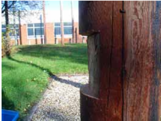
A sample damaged pole
